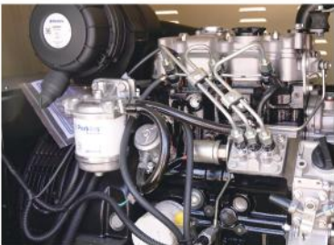
3 Cylinder Water Cooled Diesel Generator
